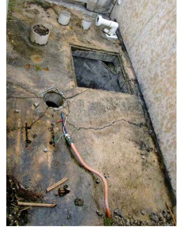
Photo No. 4 - Pump chamber No. 4 with all components stolen.
