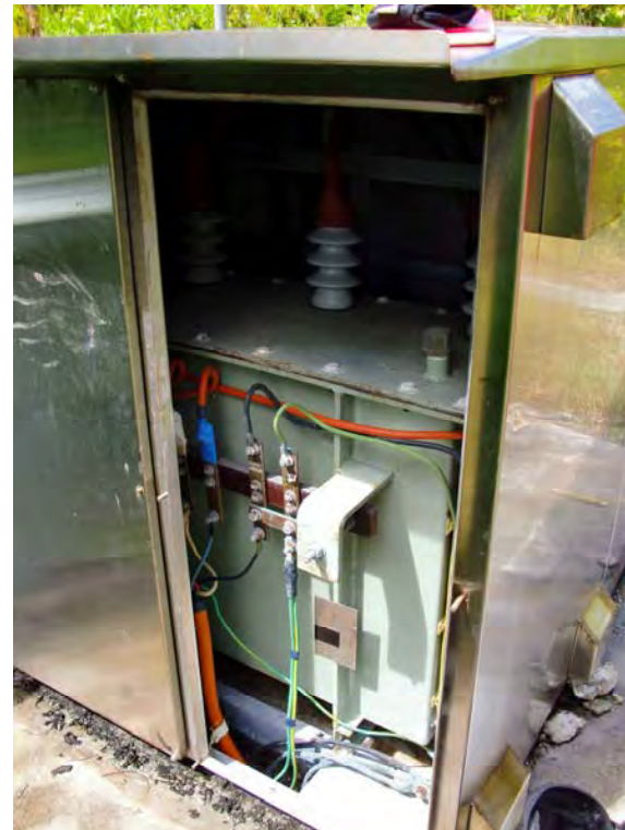
Photo No. 6 - Missing panel enabling easy access to live 11,000 volt connections.
