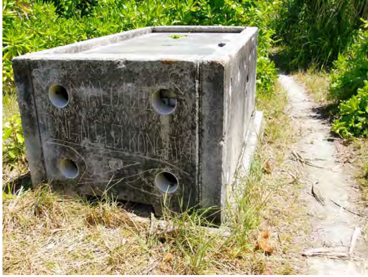
Photo No. 1 - Pump chamber No. 3 showing the large ventilation holes on the end panel.
