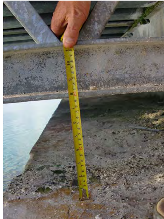
Photo No. 13 - The 200mm clearance between the lower rail and the bridge abutment.
