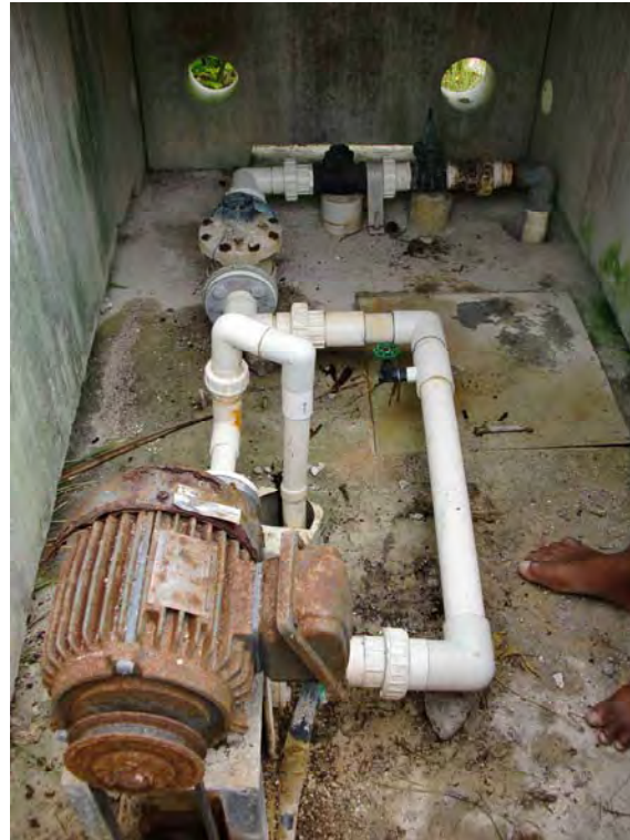
Photo No. 2 - Inside pump chamber No. 3 with complete pipework and fittings but requires refurbishment.
