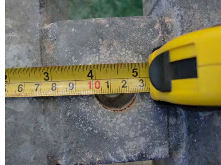
Photo No. 14 - The 25mm diameter pre-dilled hole in the lower side rail. Note the rust discolouration forming after just 6 - 9 months.
