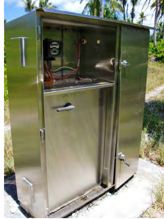
Photo No. 7 - Photo showing missing and broken door on main control unit.
