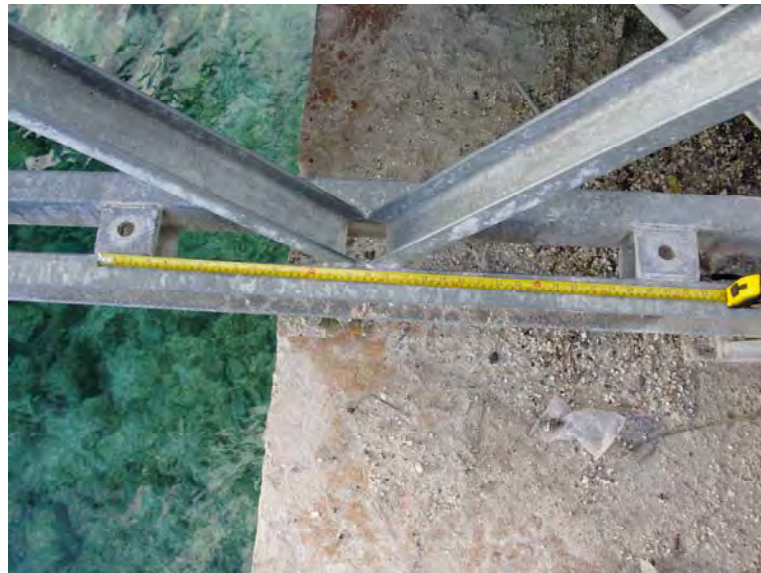
Photo No. 12 - The lower side rail is the recommended route from which the pipeline could be suspended.
