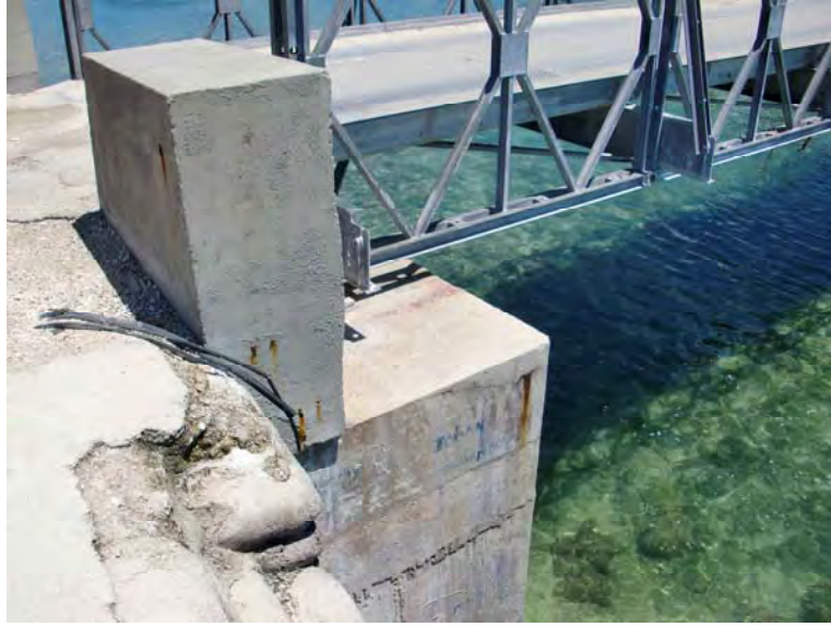
Photo No. 9 - Southern guard block which needs to be cored through or the pipe routes around. If routed around the concrete sand bags will require reinstating.
