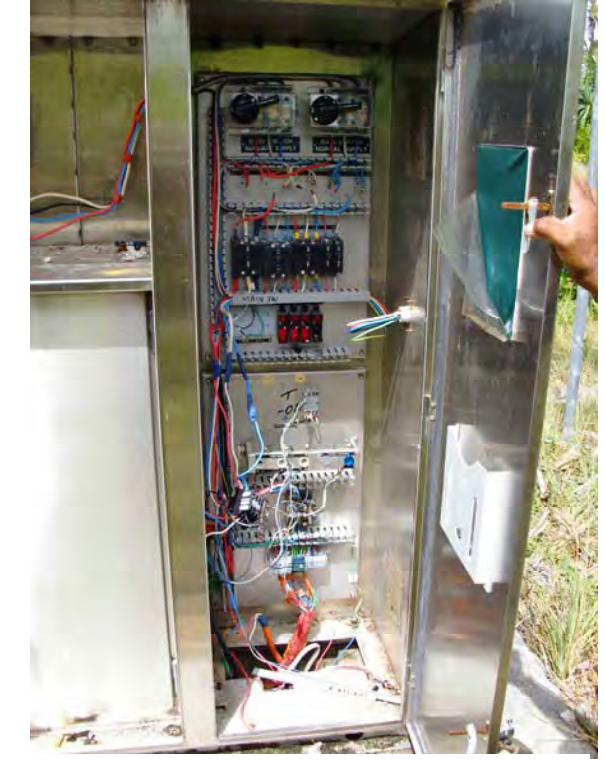
Photo No. 8 - Photo showing the vandalised electric panel due to a broken door lock on the main control unit.
