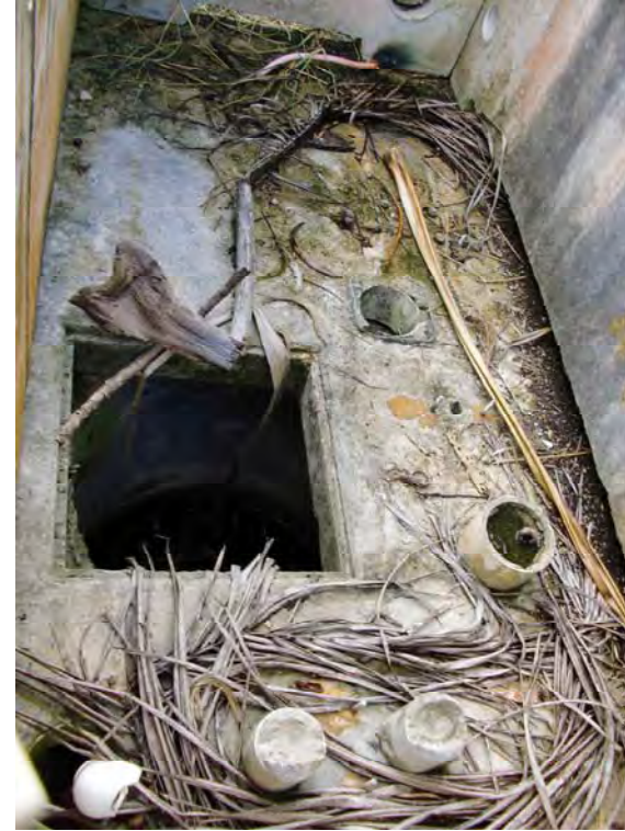
Photo No. 3 - Pump chamber No. 5 with all components stolen and vegetation has fallen into the well.
