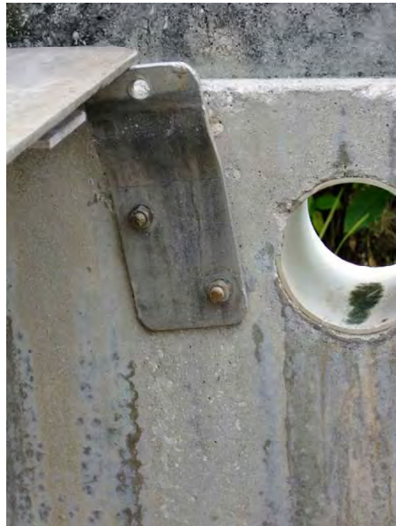
Photo No. 5 - Photo showing ease of access through chamber ventilation holes enabling the hasp bolts to be released.
