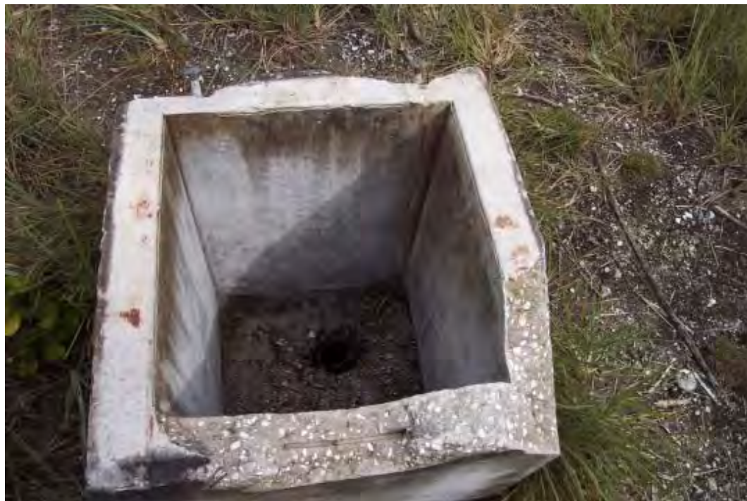
Figure 21. Vandalism to infrastructure is a reoccurring problem in water reserves. This was Bonriki salinity monitoring borehole BN4B. The steel lid has been smashed off and the piezometer tube and salinity monitoring tubes have all been removed.
