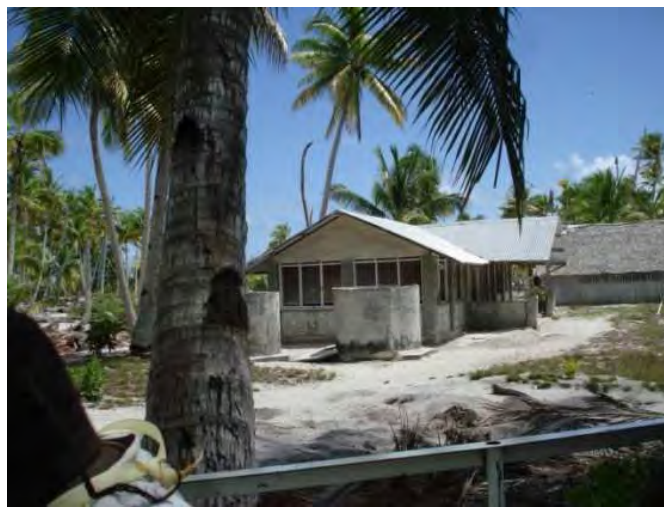
Fig.d: Tebikerai Primary School defunct concrete water tanks
