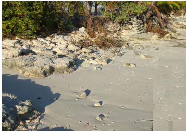
Fig. 2q: Damaged seawall, (photo by Temakei Tebano)
