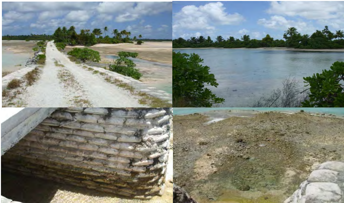
Fig.2d: Views at Teibo Causeway (from top left to right). View across causeway; accretion on lagoon side; one of five culverts; accretion on one side of culvert (photos by Temakei Tebano)
